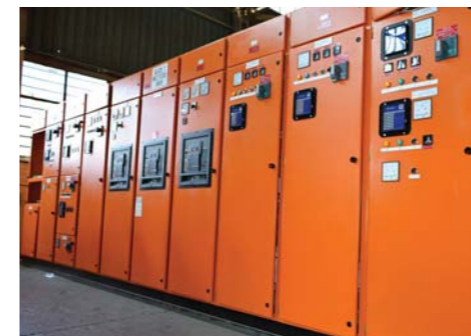
SC100 Motor Control Centre
